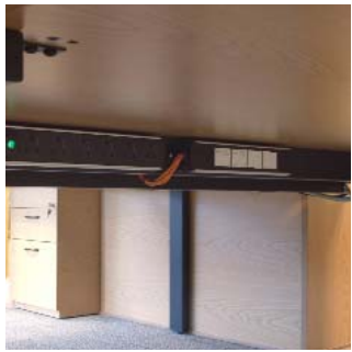
Cable managed beam
